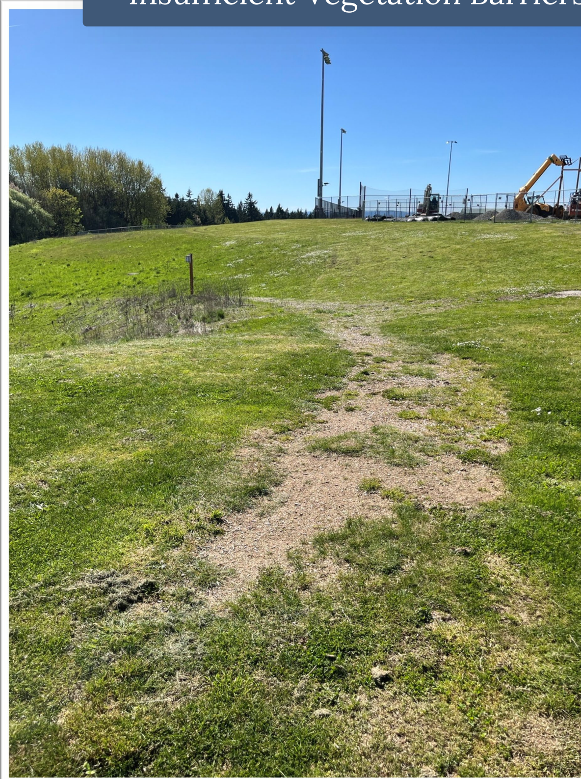
Insufficient Vegetation Barriers
