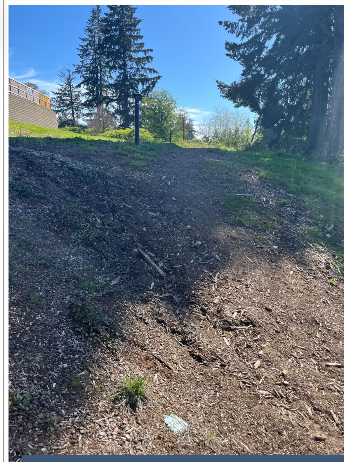
Poor Water Drainage / Steep Grade
