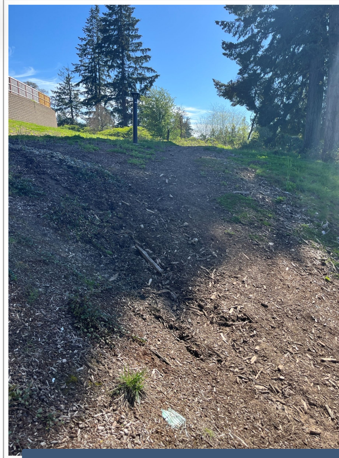
Poor Water Drainage / Steep Grade
