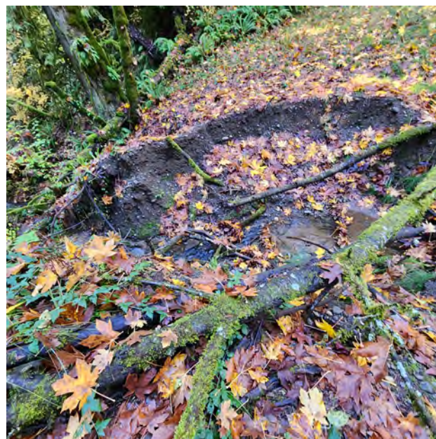
Photo 32. Large washout of logging road berm (facing west).
