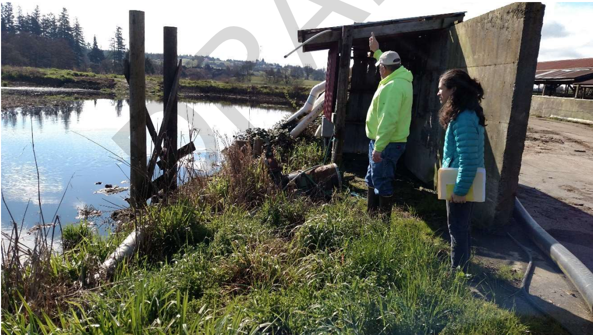
Photograph 9 – Dairy lagoon pumping station (lagoon watering).
