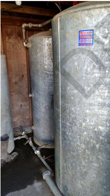
Photograph 5 – Kennedy Farms pressure tanks.
