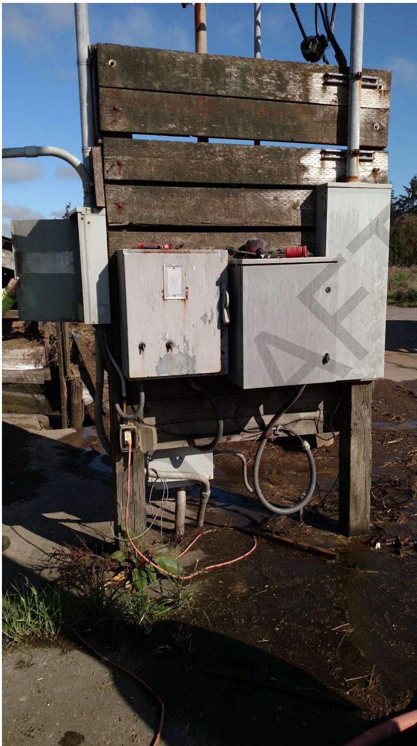
Photograph 10 – Service electrical panels for lagoon and groundwater.
