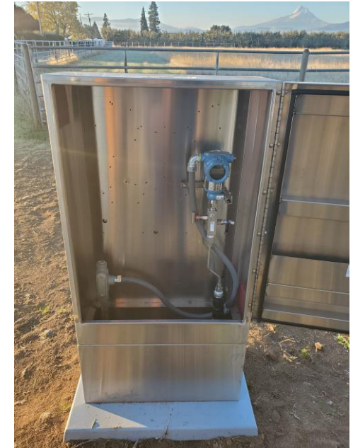
Similar Pressure Transmitter and Stand Design in Field (cabinet open)
