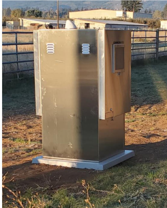
Similar SCADA Telemetry Cabinet in Field.
