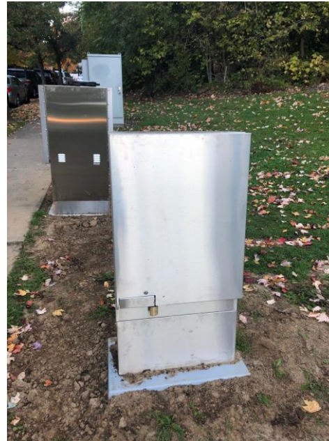
Similar Pressure Transmitter and Stand Design in Field (cabinet closed)
