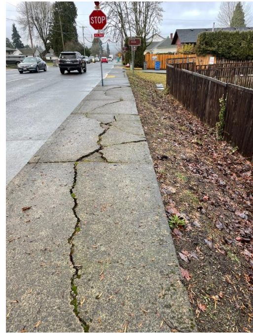
Figure 11: A Cracked Sidewalk in Downtown Ridgefield.
